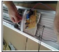
8 Fourth step: the connection cable through the back of the PCB box.
