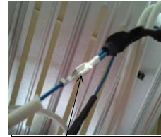
15 After removed the black silicone,see the terminal block.
